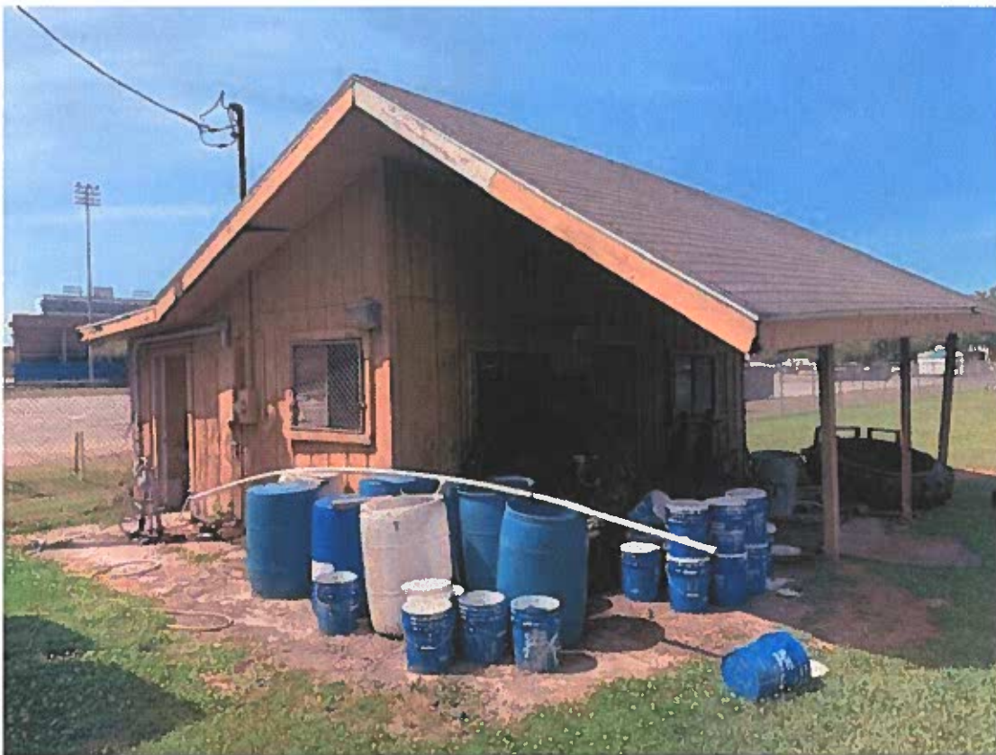
Southeast View of Football Service Building – McNeese State University, Lake Charles LA
